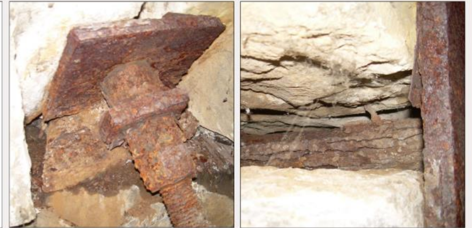
Example of the corrosion effecting the gudgeon anchor assembly at Gates 2, 3, and 4.
